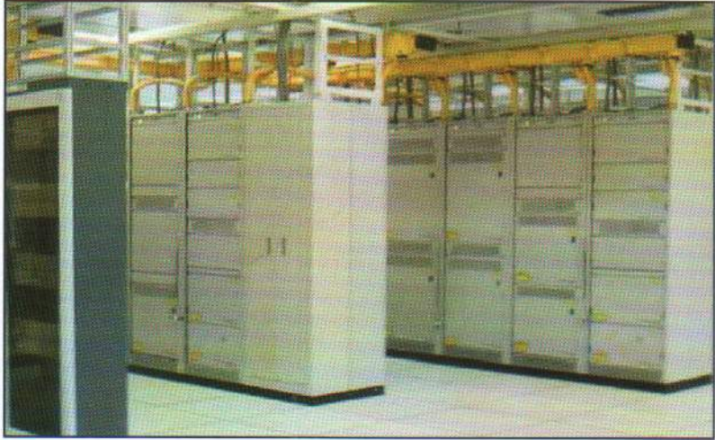
Landing station Equipment Room
