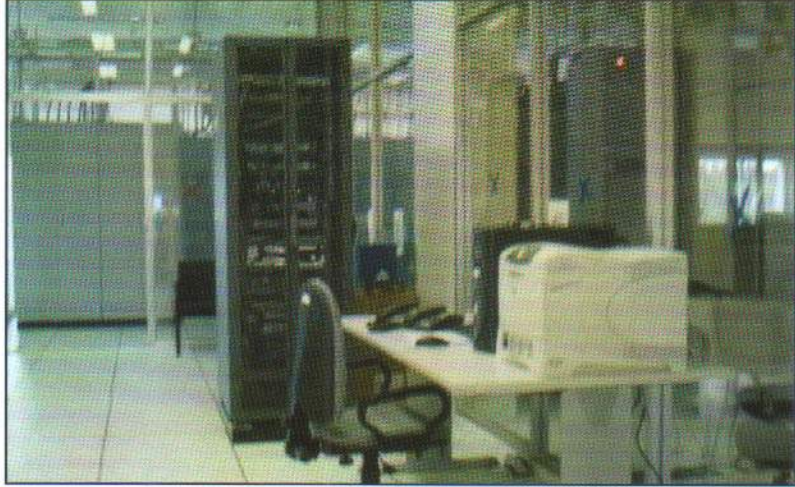
Landing station NMS Room
